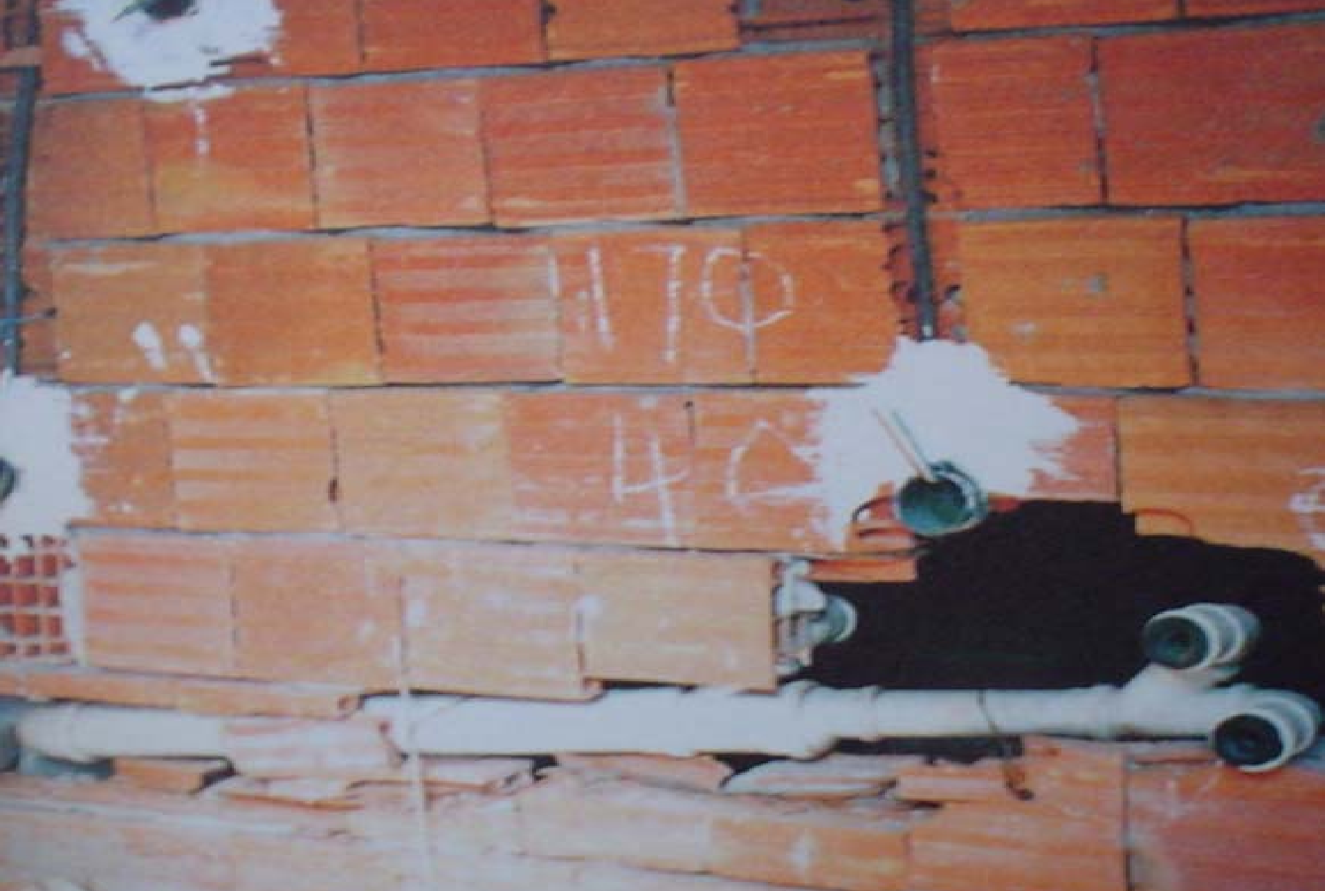
Example of imperfect planning of construction
